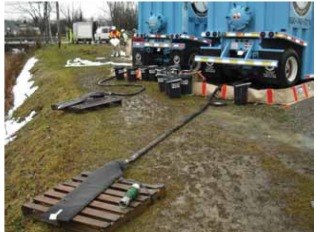
Multiple EVACs used in Wellington, OH to filter frac tank water.
