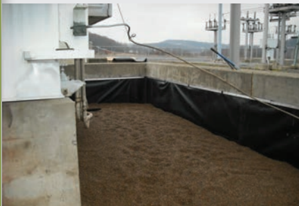
Retrofitting an old cracked concrete containment with C.I. Agent Geomembrane saved the customer time and money.
