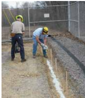
5. Optional: Granular Bentonite® can be placed in the trench to form a seal between the ground and the Barrier Boom.
