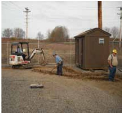
2. Dig a trench around the perimeter of the substation. Depth and width depends on your particular application of Barrier Boom. For this method, the Barrier Boom must be below grade level.
