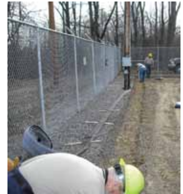
3. Inside the trench, string a line from one side of the trench to the other to keep the stakes and Barrier Boom straight.
