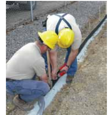
6. Stand the Barrier Boom up against the stake and staple or screw near the top of the Barrier Boom. If using rebar, lean Barrier Boom against it. Black fabric side to face the inside.
