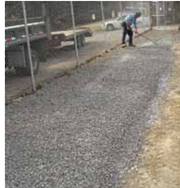
10. Cover area with clean stone and rake until the Barrier Boom is completely covered.
